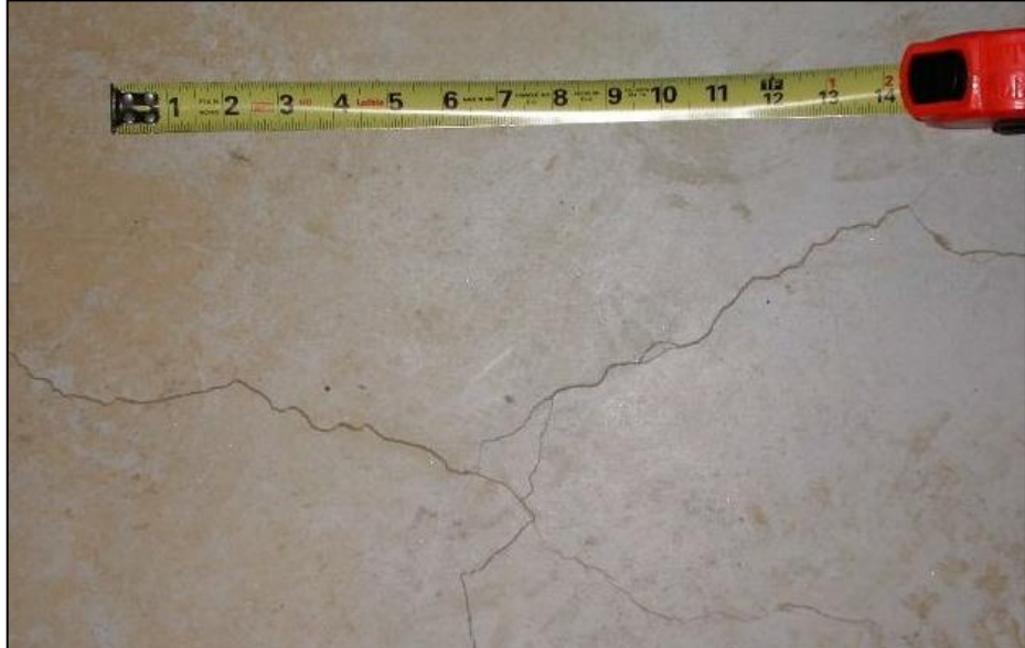
Figure1.9 Minor cracks on floors of ground floor
